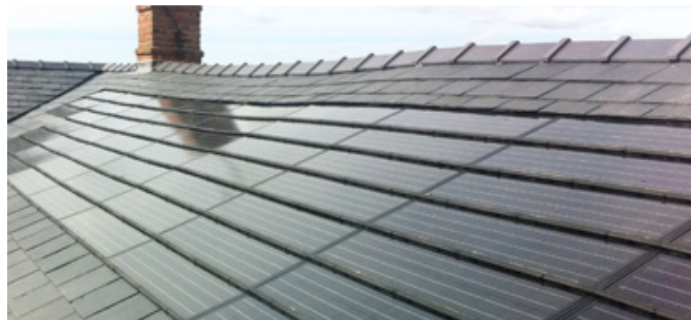
Solar PV system (C21e slate)
